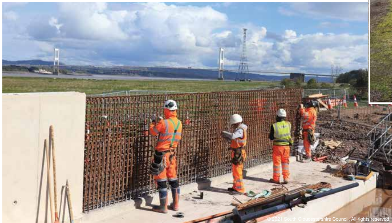
Above: Raising the outfall structure at Cake Pill. Below Left: Ongoing flood defence work at Severn Beach North. Below Right Installation of concrete flood defence wall at Aust Wharf Road.
