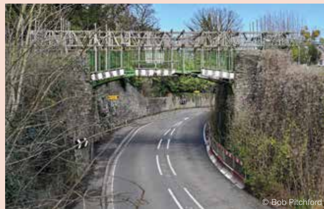
After the Damage.
