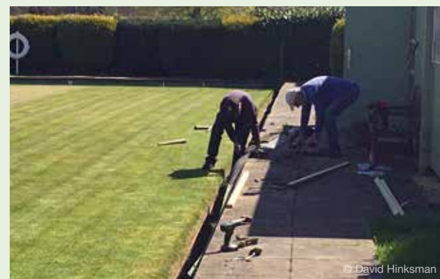
Phill and Alan carrying out repairs to the green ahead of opening day on April 10th.
